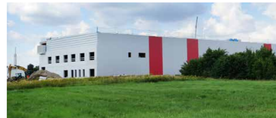
Taking shape: Building work on the new factory for Wefo-tec Deutschland GmbH in the Markendorf Business Park in Frankfurt (Oder) is progressing according to schedule. Construction of the first production hall should be completed by the end of the year. As soon as this is ready, construction of the second factory hall is due to commence while, at the same time, preparations are already underway for the start of production operations.
